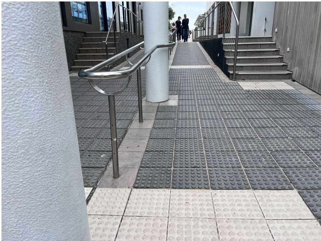
An example of how NOT to use Tactile Ground Surface Indicators
